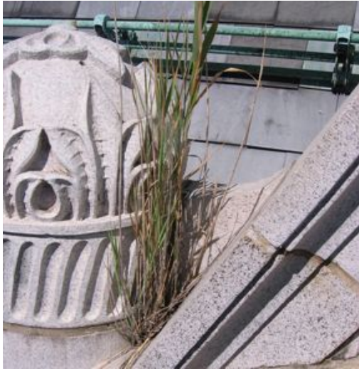
Unintended “living walls”: vascular plant growth in terra cotta
