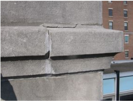
Horizontal and vertical displacement in limestone
