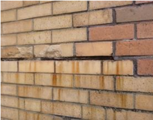
Pack rust in a relieving angle causing adjacent brick to spall
