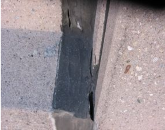
Failed sealant at an expansion joint in precast concrete panels
