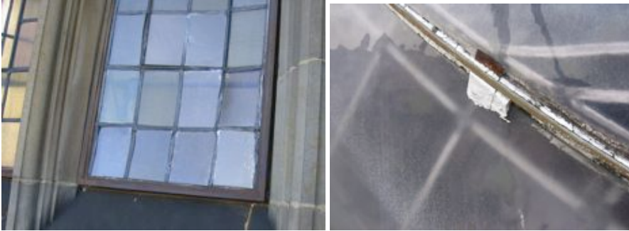
Bulged glass panes in a multi-light window Putty failure in window glass
