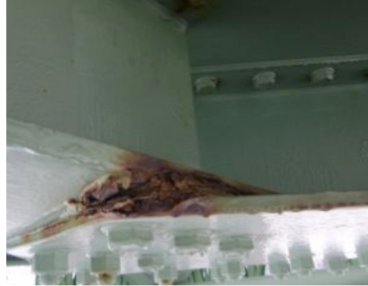
Pack rust between steel plates of a bridge truss
