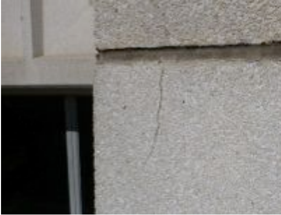
Incipient spall in concrete
