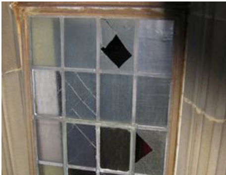
Cracked, loose and missing glass in a multi-light window
