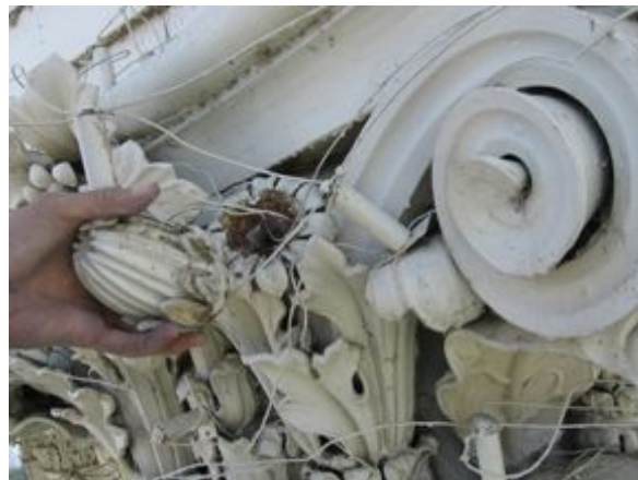
Unsecured cast iron ornament
