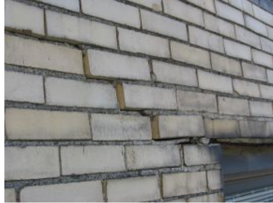
Horizontal and vertical displacement in brick
