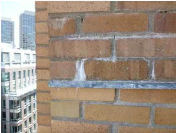
Leached salts at mortar joints in brick
