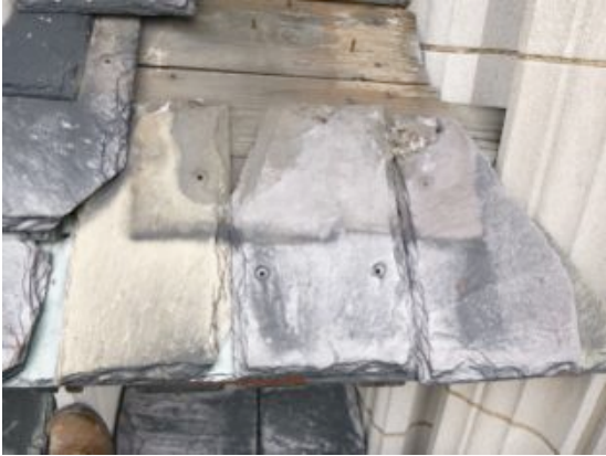
Failed fasteners and missing slates
