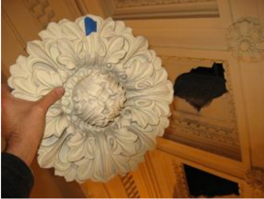
Unsecured plaster medallion
