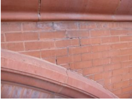
Crack system through joints in brick
