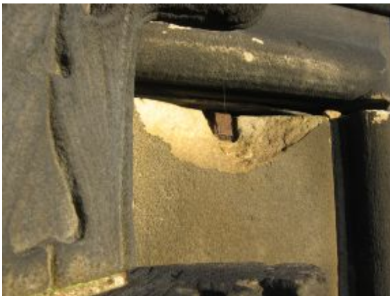
Cramp spall in limestone due to rusted steel anchor
