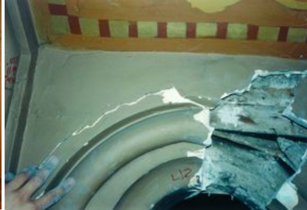
Water-damaged plaster that has separated from the substrate
