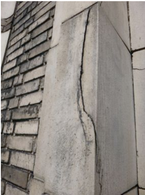
Severe crack through a terra cotta unit
