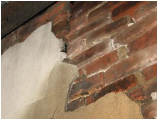
Unsecured stucco separating from the brick substrate
