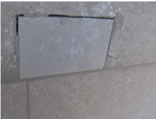
Failed dutchman repair in limestone
