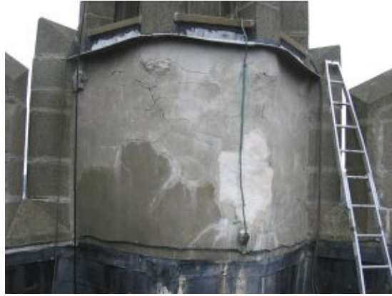
Failed crack and patch repairs in stucco
