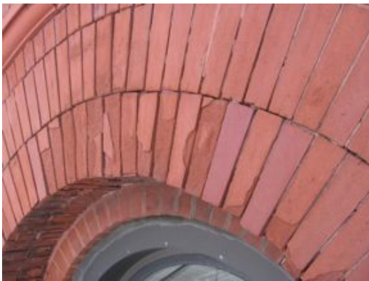
Face-spalled brick, above
