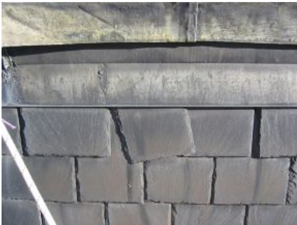
resulting from a failed fastener
