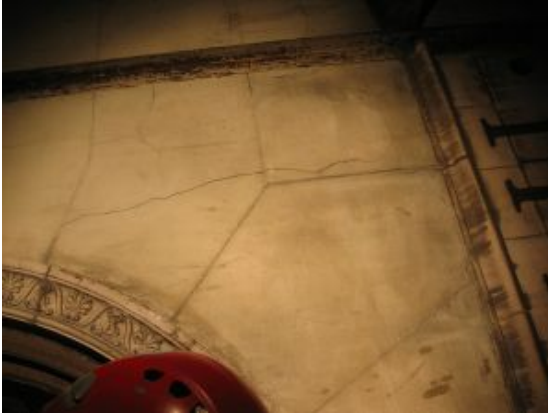
Cracks through stucco scored to imitate stone masonry
