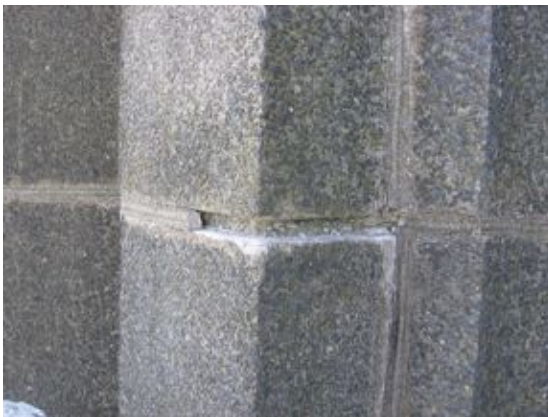
Failed mortar in cast stone masonry
