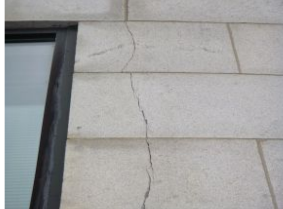
Crack system through units in granite
