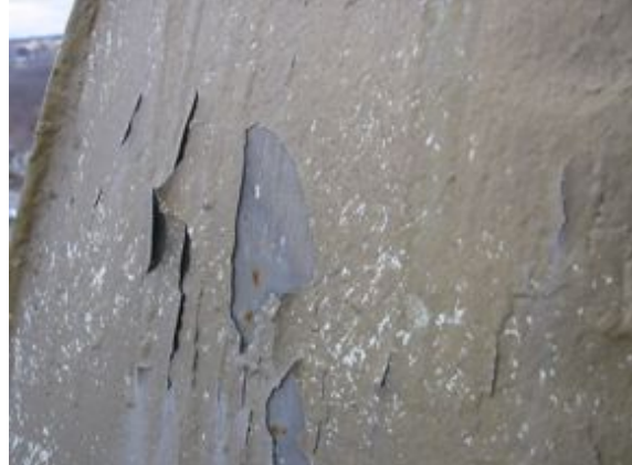
Failed paint coating on sheet metal
