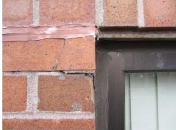
Bonded brick spall held in place by sealant
