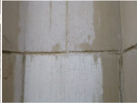
Efflorescence in cast stone
