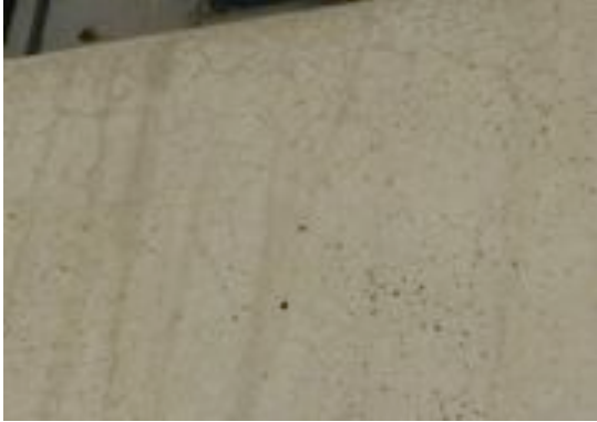
Crazing in concrete
