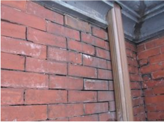
Missing mortar in brick masonry
