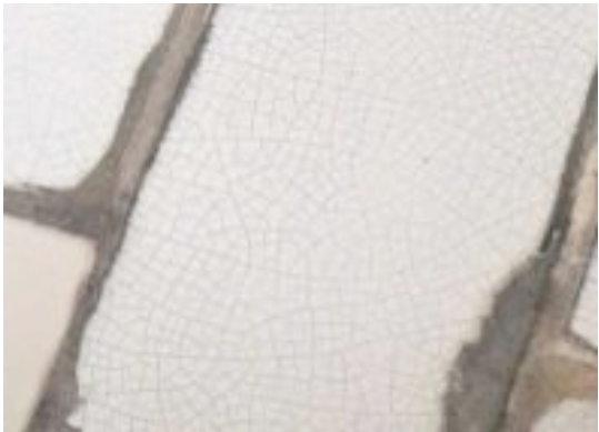
Crazing in a glazed terra cotta tile
