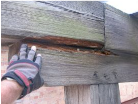
Structural wood members exhibiting biological growth (algae) and rot
