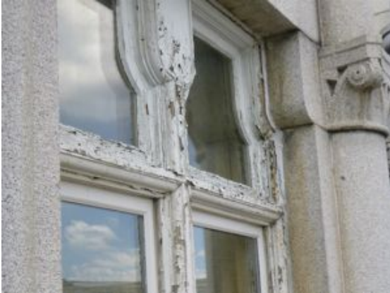
Failed paint coating on wood
