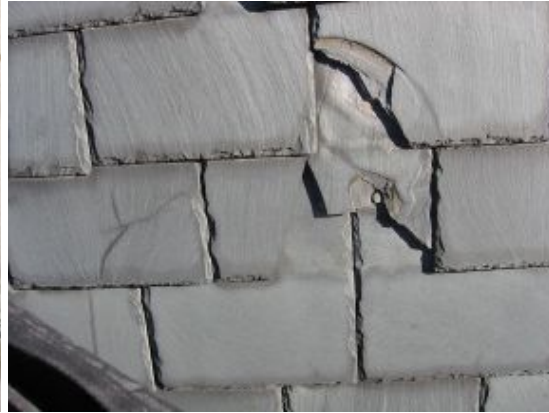
Cracked and missing slates
