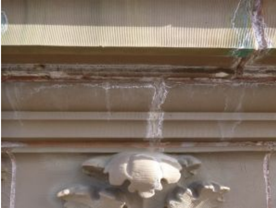
Leached salts in terra cotta
